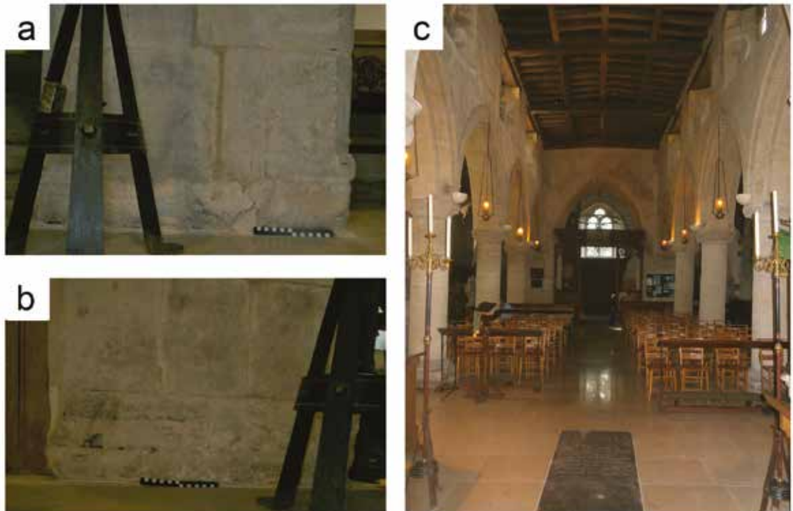
FIGURE 6 Bases of jambs of chancel arch (a) north jamb (b) south jamb; (c) Nave looking west
