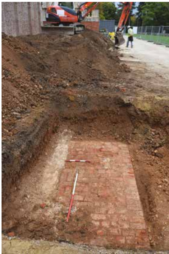
FIGURE 14 East-west plinth type wall exposed in front of western half of terrace
