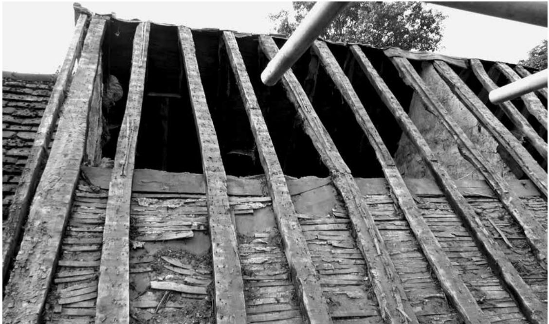
FIGURE 6 Rafter structure of 3 High Street (1550s) showing common rafters set at same height as the principal rafters. Note typical use of curved windbraces.
