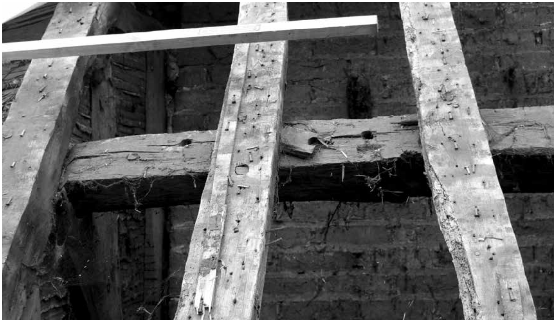
FIGURE 7 Oak pegs used to secure the rafters to the backs of the purlins (3 High Street)
